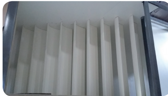
Figure 26. Turning-vanes mounted in the corner C1.
